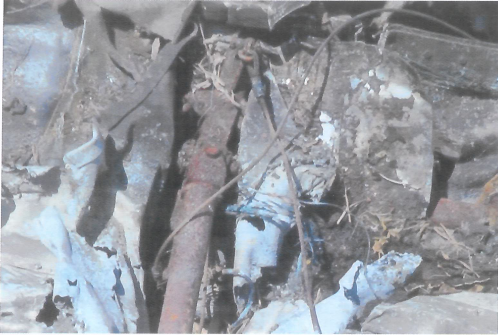
Photo 11 : Elevator end connections at the height of the control stick
